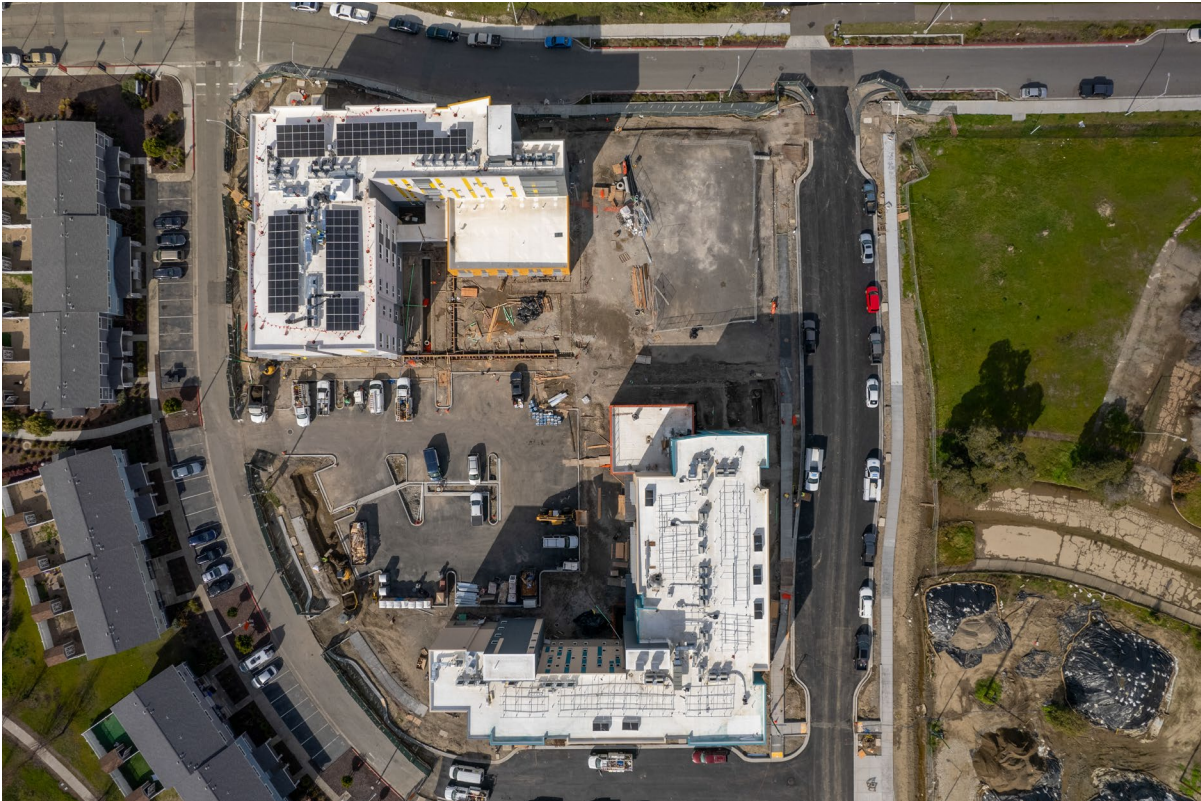
Aerial view looking down on NH Block A showing roof tops and exterior grading work.
