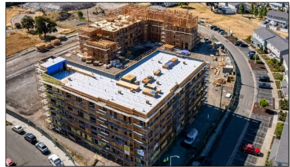
1. Active construction of The Estuary I and Linnet Corner as of July 2024.
